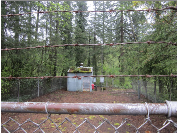
Photo A. Existing NW Natural facility.
