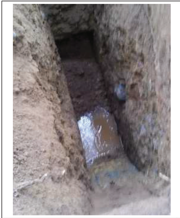
Groundwater Seeps at 10 feet in TP-1
